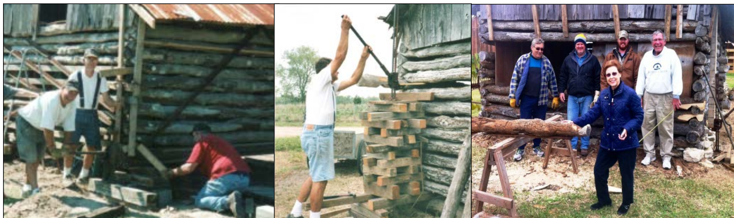
Vasek Brothers: Ernest, Ed and David hard at work. Center: Ed Vasek leveling one log at a time. Right: Restoration was needed by 2014. Mary Vasek oversaw the repairs with volunteers Harry King, Dan Bolton, Corie Bolton, and Ernest Vasek. Bottom left: The log crib pictured in the stained glass window created by John Keble.
